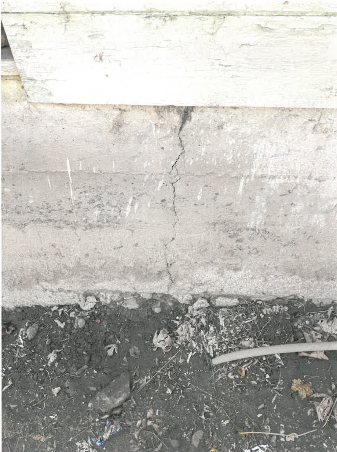
FIGURE 2: VERTICAL FOUNDATION CRACK AT EAST SIDE OF STRUCTURE FOUNDATION, LIKELY CAUSED BY EXPANSION AND CONTRACTION OF THE CLAYEY SOILS DUE TO PRESENCE OF WATER.
