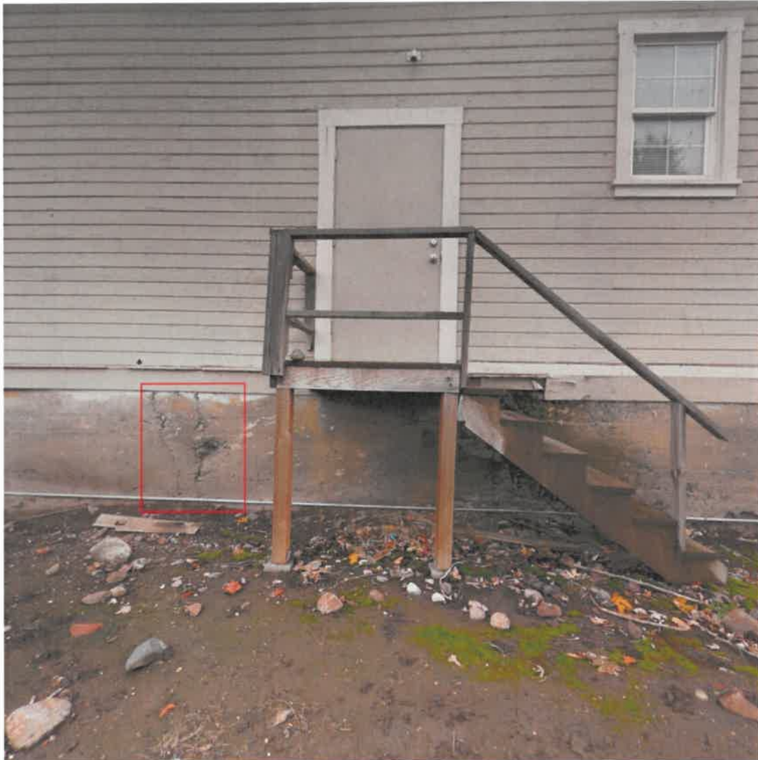
FIGURE 9: STAIRWELL AT EAST SIDE OF STRUCTURE LEADING TO THE MAIN HALL THAT IS RECOMMENDED TO BE REPLACED. THE RED BOX LOCATES AN AREA WITH POOR CONCRETE, WHICH HAS CAUSED SIGNIFICANT LOSS OF CEMENT AND LOAD-CARRYING CAPACITY.
