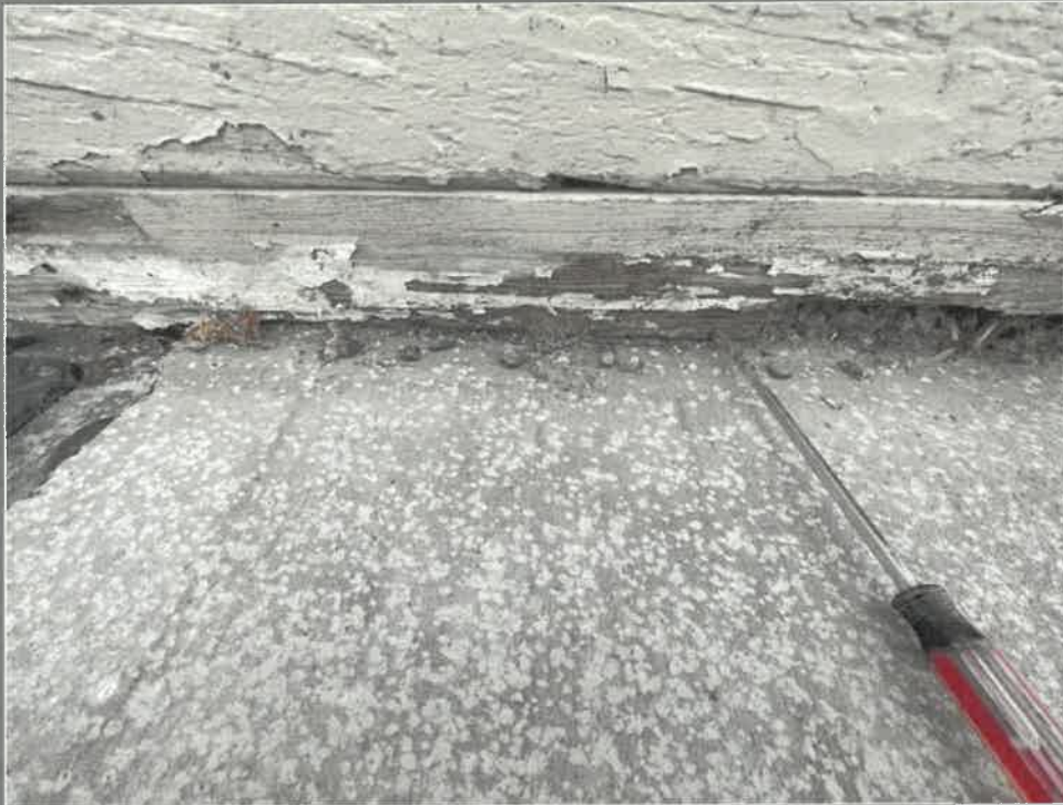
E. Item 1(Picture) Wood decay at sidewalk
