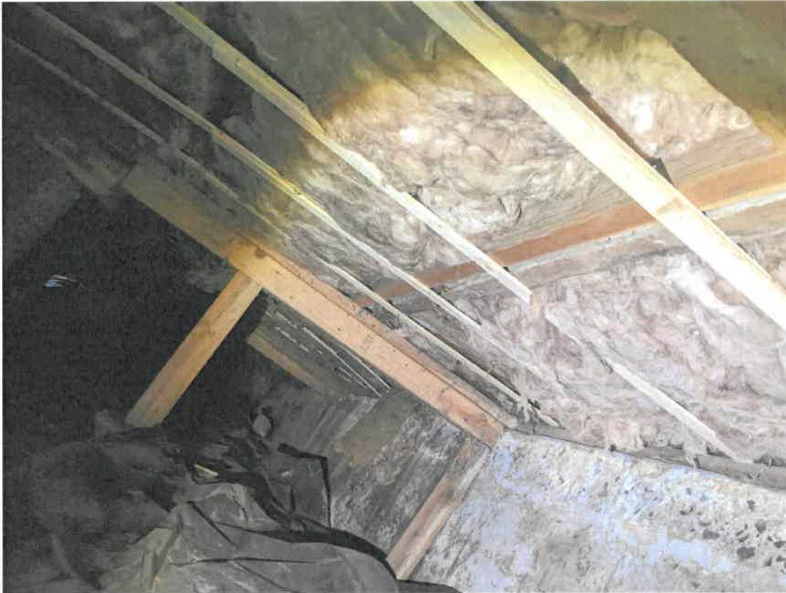
FIGURE 16: DOUBLE 2X8 FLOOR JOIST AT NORTH END OF STRUCTURE WHERE ONE IS CLEARLY DAMAGED (RIGHT). THIS SUGGESTS THAT DOUBLED JOISTS MAY NOT BE ORIGINAL, BUT WERE RETROFITS TO REINFORCE EXISTING JOISTS.
