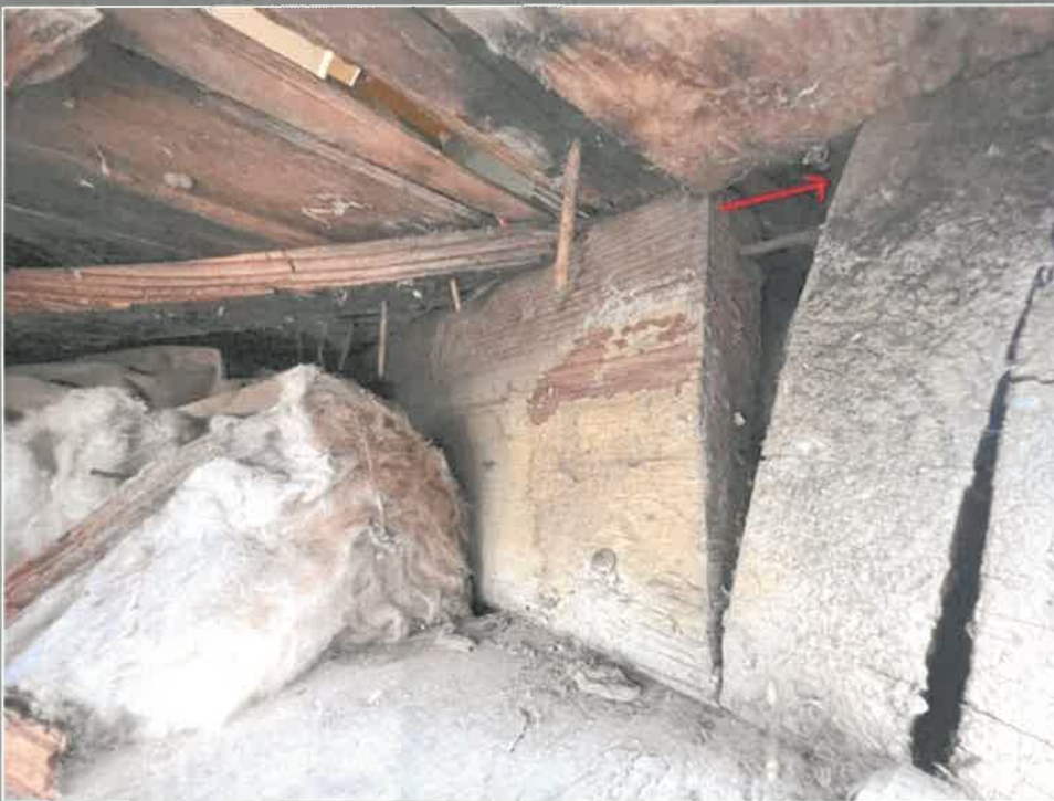
B. Item 13(Picture) As walls are pushed off the rim joist is pulling away as well. Eastern side near bottom plate bulge
