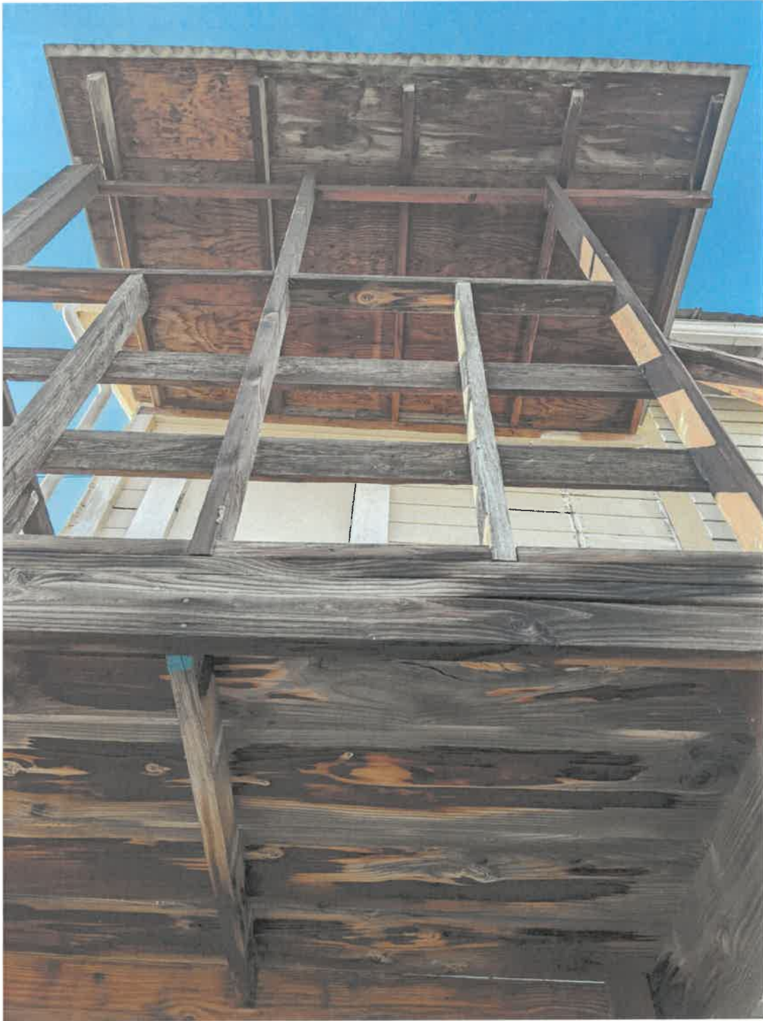
FIGURE 7: THE RAILING SYSTEM AT THE SOUTHEAST STAIRWELL DOES NOT MEET CURRENT CODE REQUIREMENTS.
