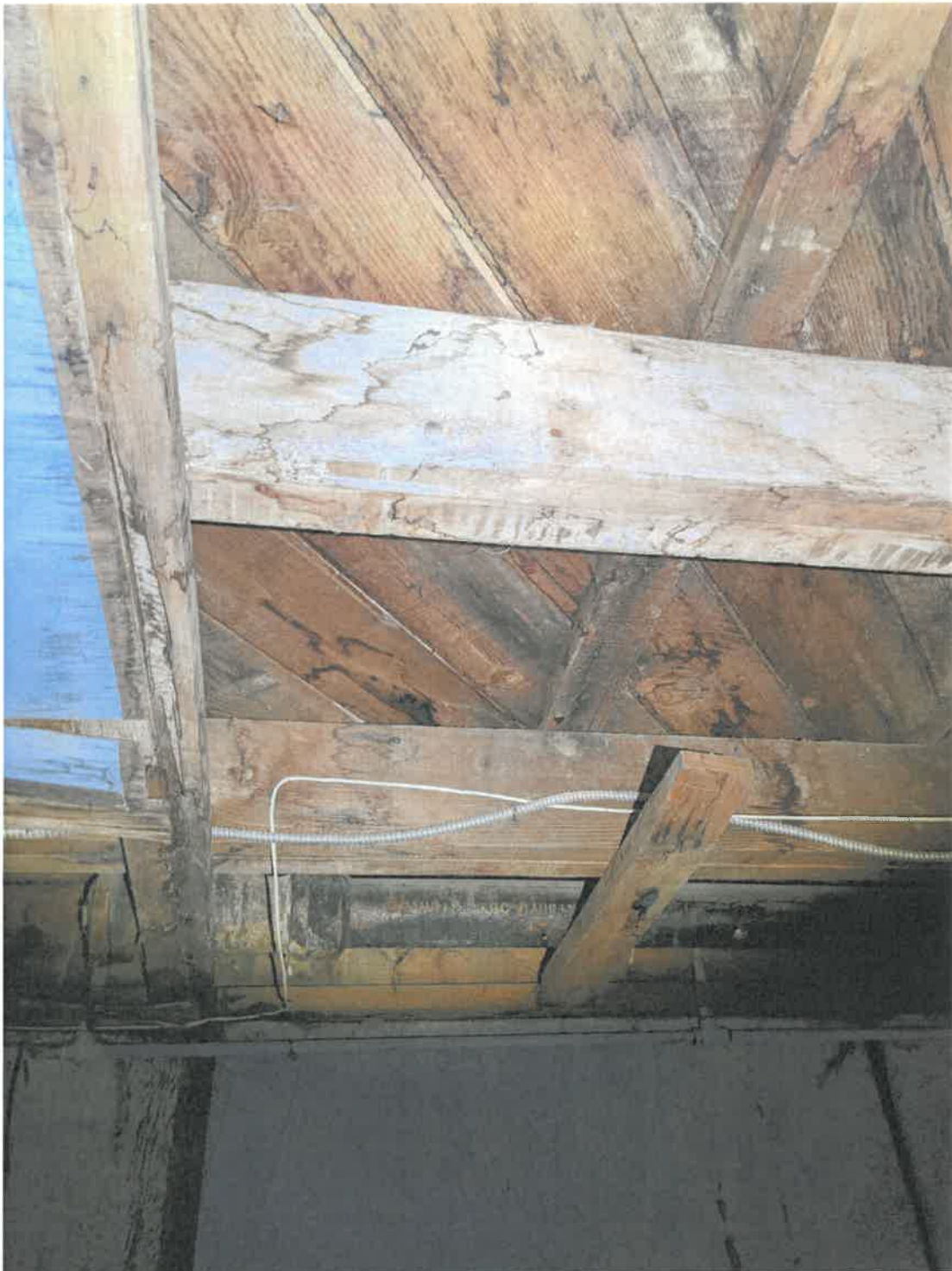
FIGURE 18: WATER DAMAGED DOUBLE FLOOR JOISTS WITH DIAGONAL TONGUE AND GROOVE ABOVE TO SUPPORT THE STAGE (FACING EAST).
