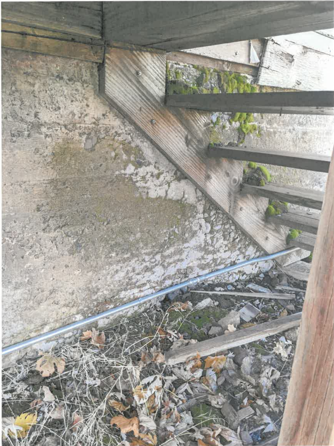
FIGURE 8: PLANT GROWTH AT THE STAIRWELL SUGGESTS MOISTURE PRESENCE, WHICH CAN LEAD TO WOOD DECAY.
