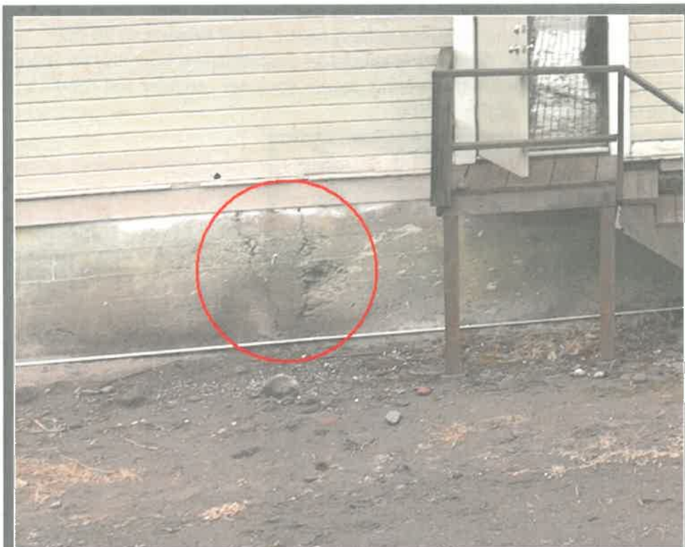
A. Item 10(Picture) Shear cracking at exit door
