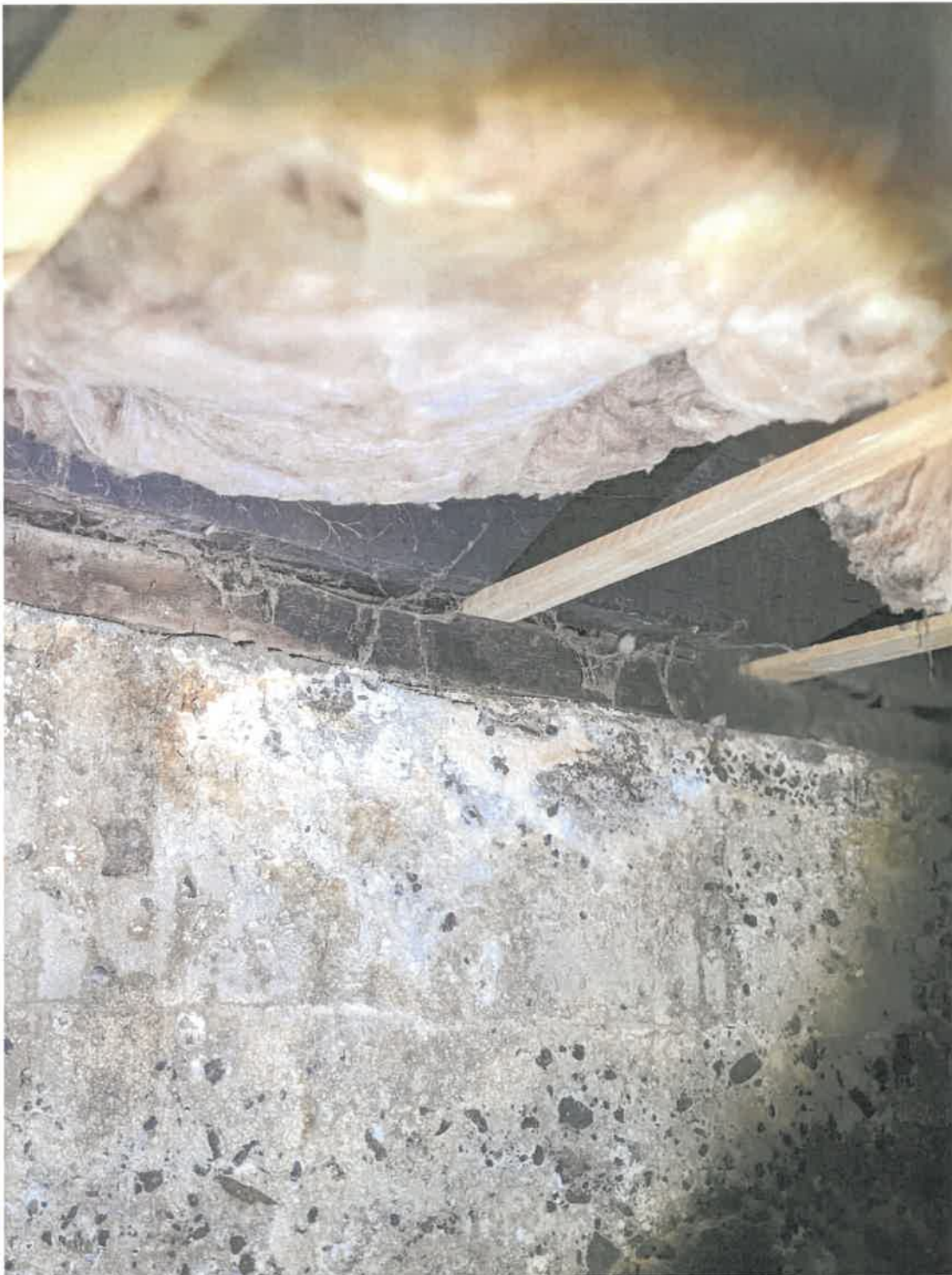
FIGURE 20: CLOSE-UP OF CHARRED RIM JOIST LEFT IN PLACE. IT IS RECOMMENDED TO REMOVE AND REPLACE THIS ELEMENT.
