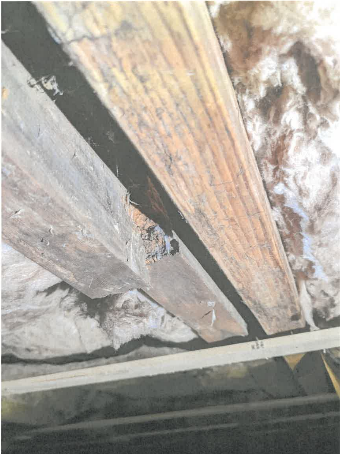
FIGURE 22: NOTCHED OR DAMAGED JOIST (LEFT) REINFORCED WITH NEW JOIST (RIGHT).
