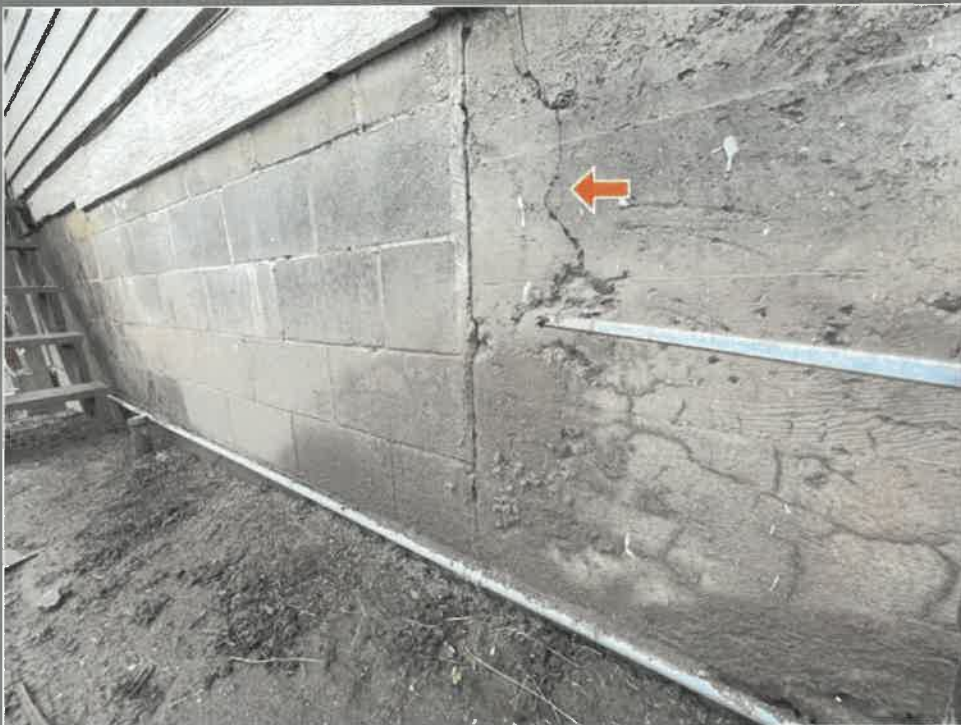
A. Item 4(Picture) Cracking at corner of original building
