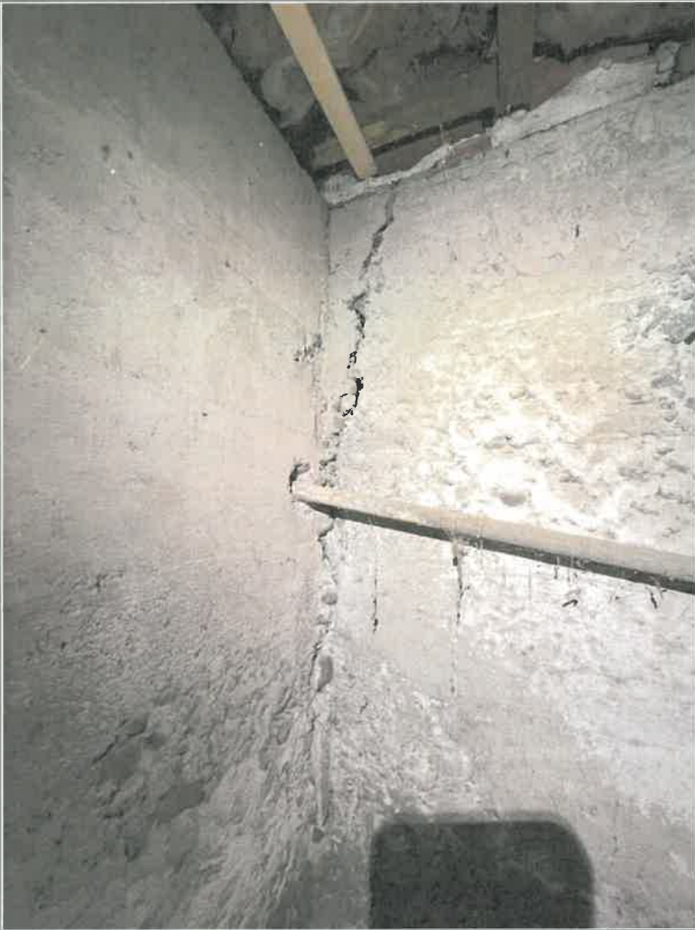
A. Item 5(Picture) opposite side of Item 4
