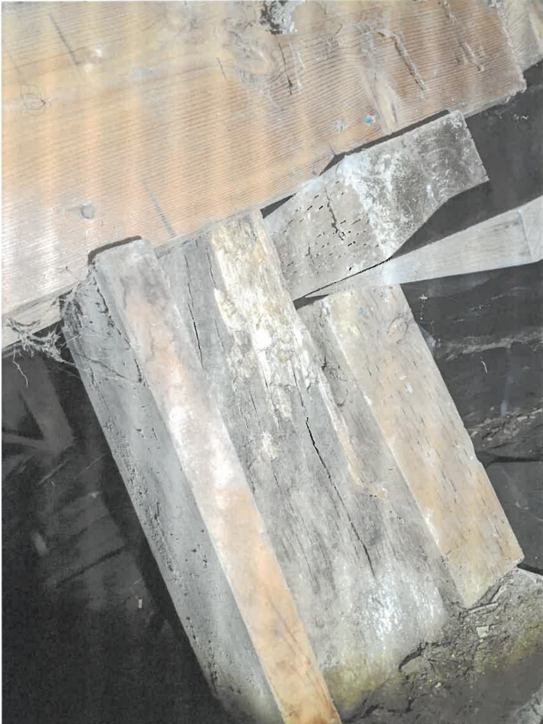
FIGURE 15: FUNGAL DECAY AT 6X6 POST IN CRAWLSPACE BELOW THE MAIN HALL.
