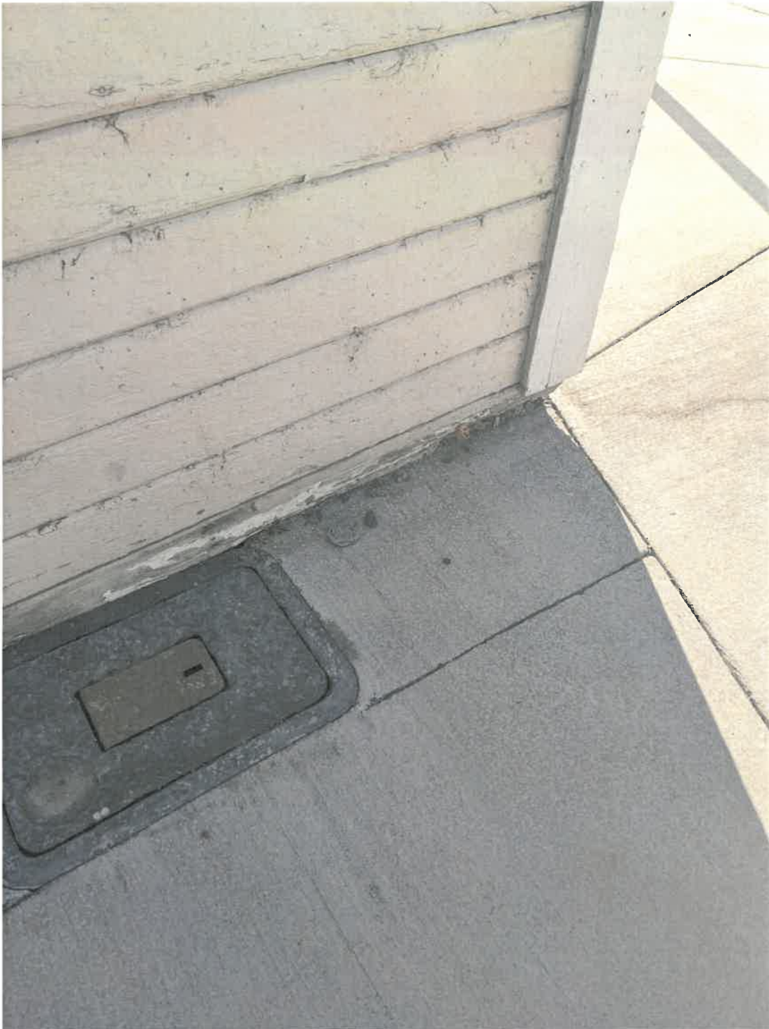
FIGURE 14: ROTTING FINISH WOOD AT NORTHWEST CORNER OF STRUCTURE, ASSUMED TO BE CAUSED BY EXPOSURE FROM MOISTURE IN CONCRETE.
