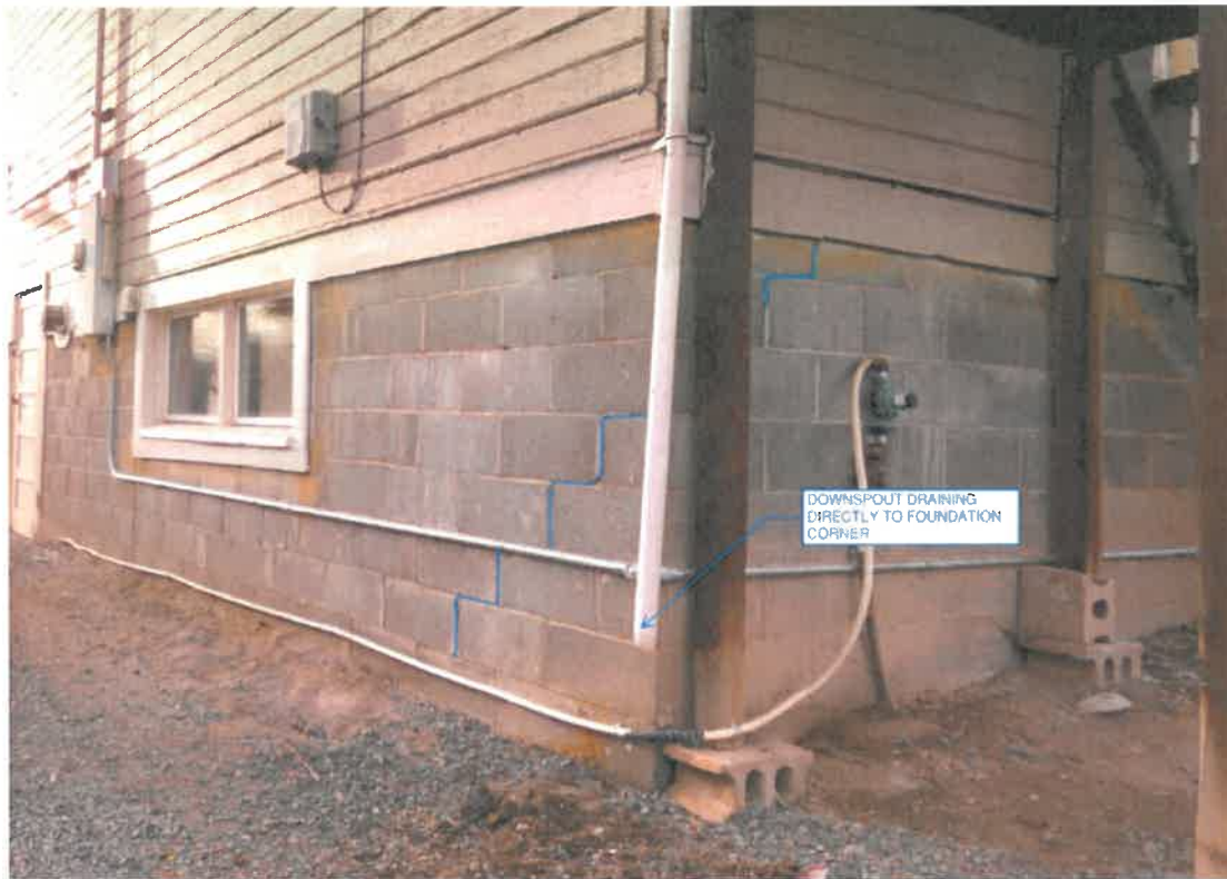
FIGURE 4: SOUTHEAST BUILDING CORNER (FACING NORTHWEST) SHOWING CRACKING DUE TO FOUNDATION MOVEMENT CAUSED BY MOISTURE FROM DOWNSPOUT.
