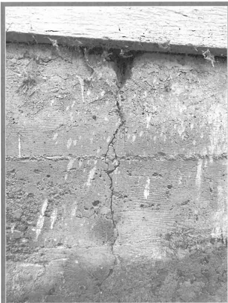
A. Item 2(Picture) Shear cracking broken foundation sliding past each other.
