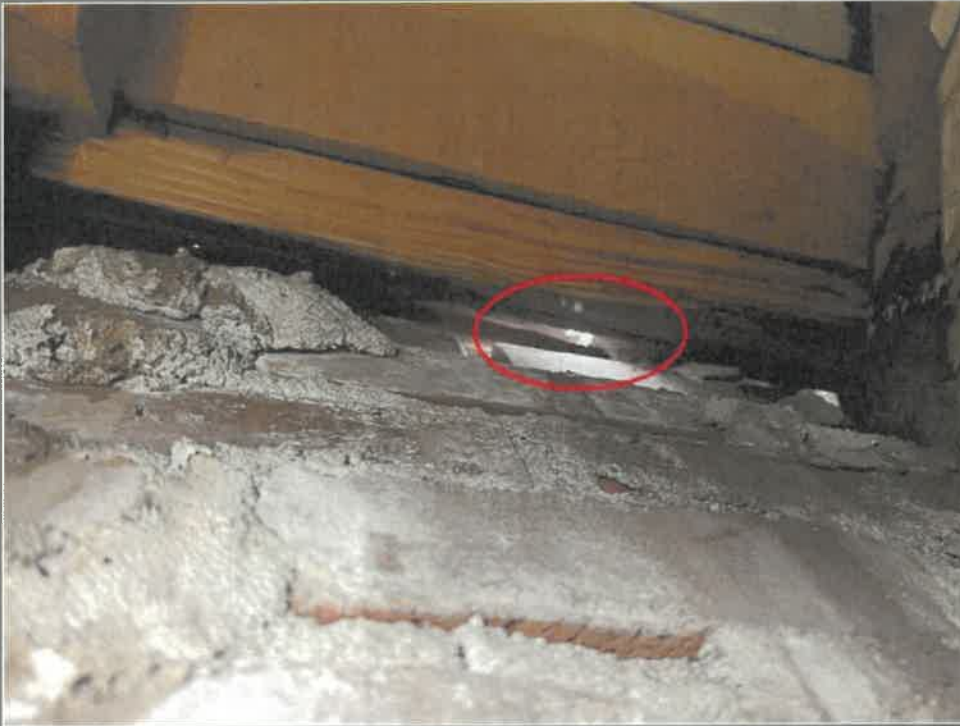
H. Item 3(Picture) Holes through flashing
