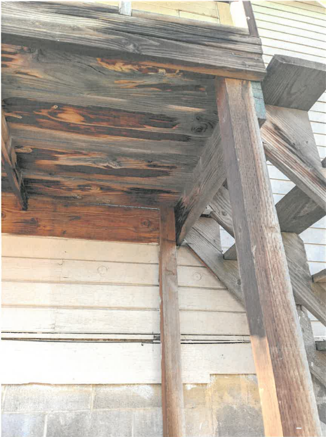
FIGURE 6: MOISTURE DAMAGE AT THE SOUTHEAST EXTERIOR STAIRWELL IS LIKELY TO LEAD TO DECAY AND ROT. THE POST CONNECTION TO BEAMS IS INADEQUATE FOR THE REQUIRED LOADING AND DOES NOT MEET CURRENT CODE REQUIREMENTS.
