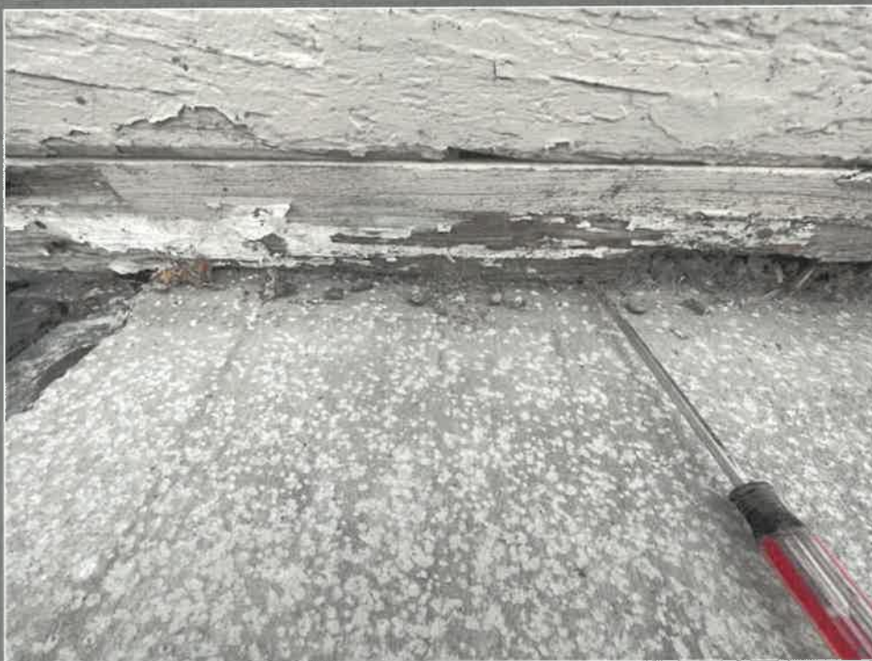
E. Item 1(Picture) Wood decay at sidewalk
