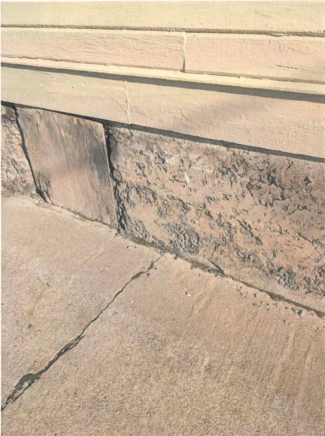
FIGURE 12: SCALING AND SPALLING AT FOUNDATION AT WEST SIDE OF STRUCTURE.
