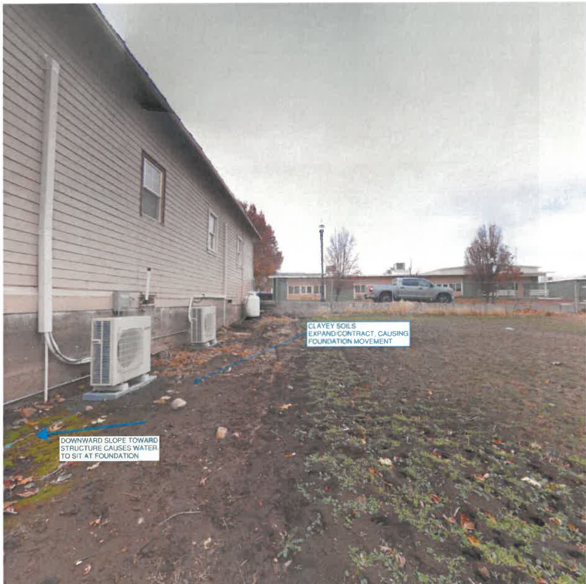
FIGURE 1: GRADING AT EAST SIDE OF STRUCTURE ATTRACTS WATER TO THE FOUNDATION, WHICH CAN CREATE VERTICAL CRACKS (FACING NORTH)
