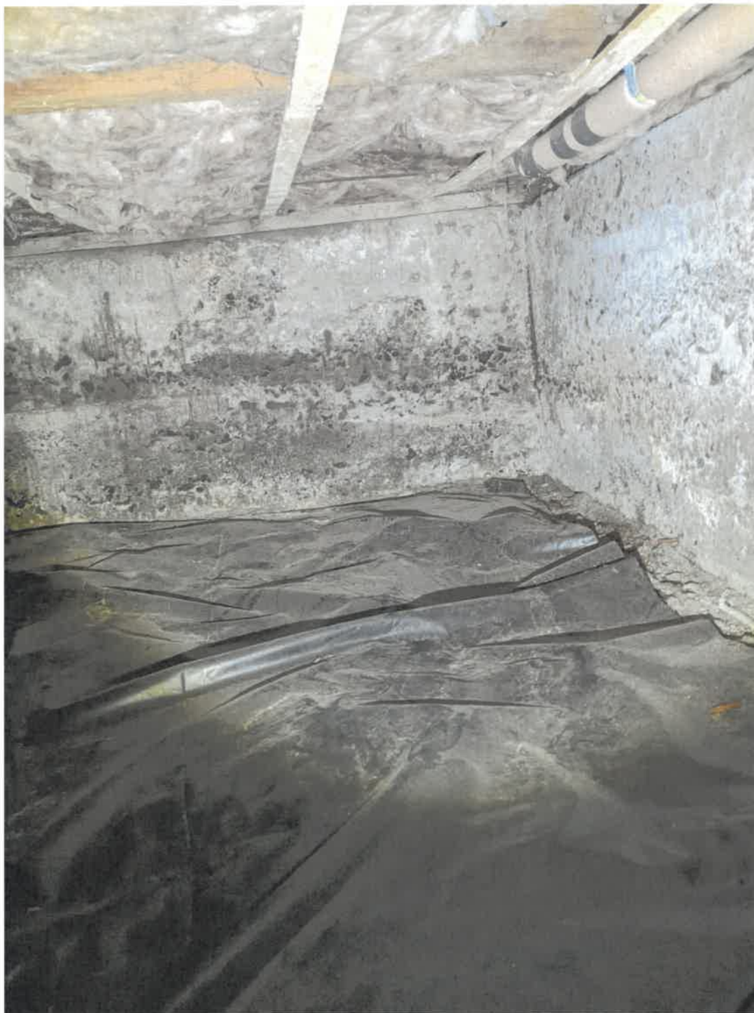
FIGURE 13: INTERIOR FOUNDATION WALL AT NORTHEAST BUILDING CORNER, SHOWING SPALLING AT NORTH END.
