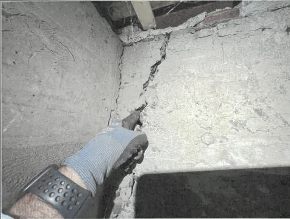
A. Item 6(Picture) Pull apart tension crack. Building pulling away to East.
