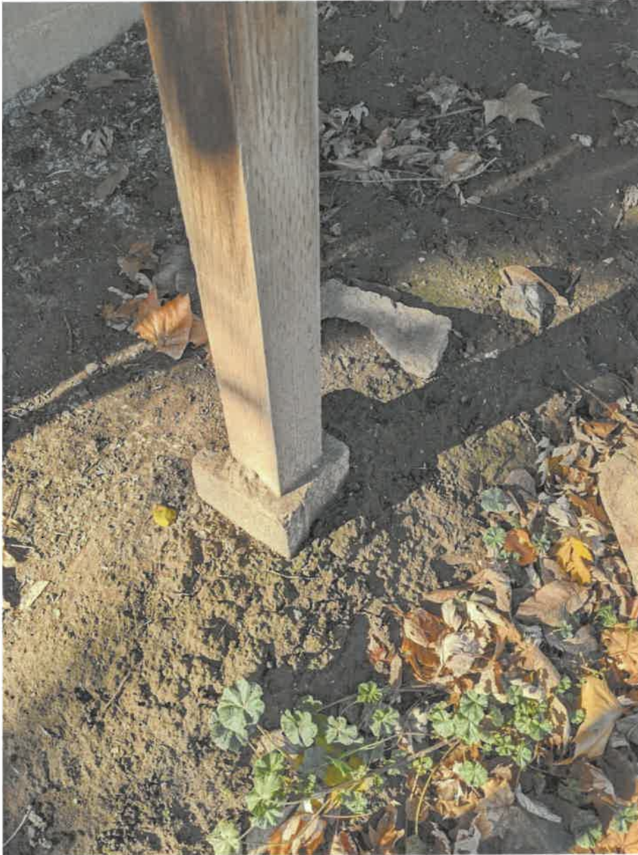
FIGURE 5: A PRESSURE-TREATED 4X4 POST AT THE SOUTHEAST STAIRWELL SERVING THE 1940S COSTUME ROOM ADDITION, SITTING UNCONNECTED TO A CMU BLOCK FOOTING. THIS CONDITION IS CONSIDERED UNSAFE.
