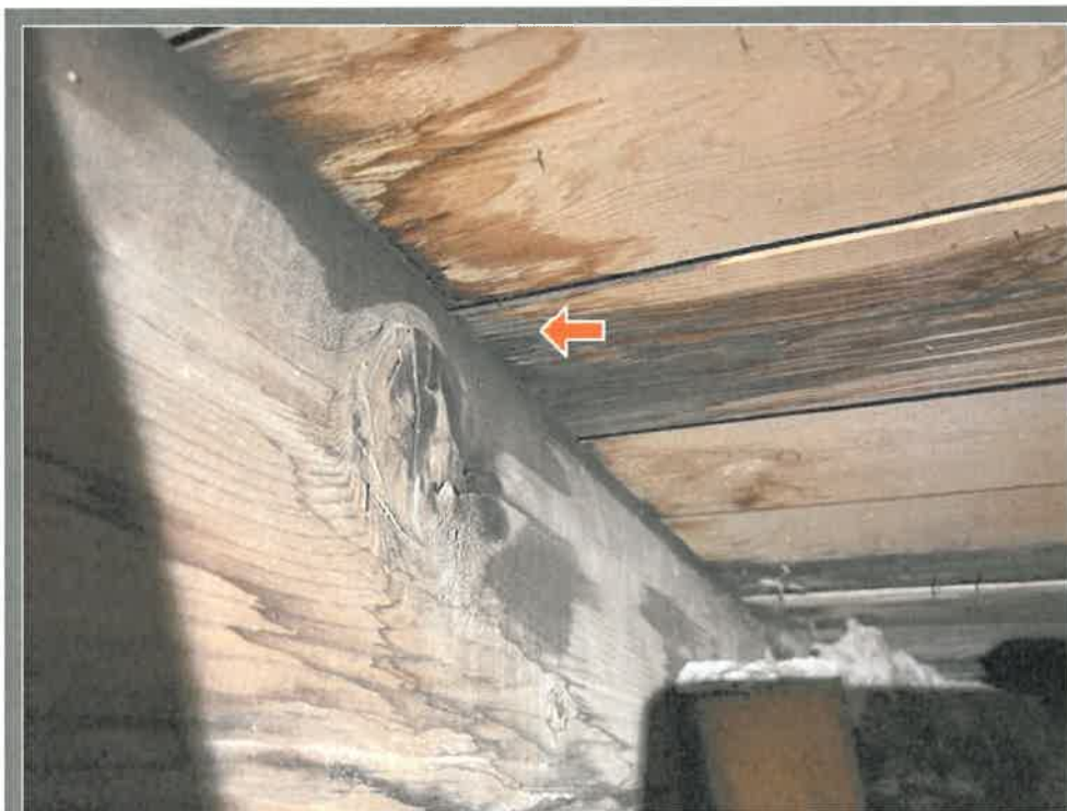
H. Item 2(Picture) Moisture damage from rusted flashing
