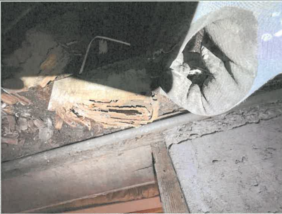
B. Item 19(Picture) In crawlspace wood debris was prevalent under vapor barrier and above.
