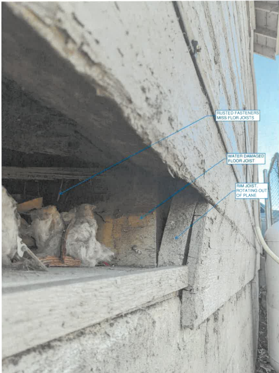
FIGURE 23: EAST WALL AT MOST SEVERE LOCATION OF WALL MOVEMENT. THE RIM JOIST WAS NOT INSTALLED TO THE SHEATHING TO RESIST IT FROM ROTATING OUT-OF-PLANE, CAUSING THE WALL TO PULL AWAY FROM THE STRUCTURE.
