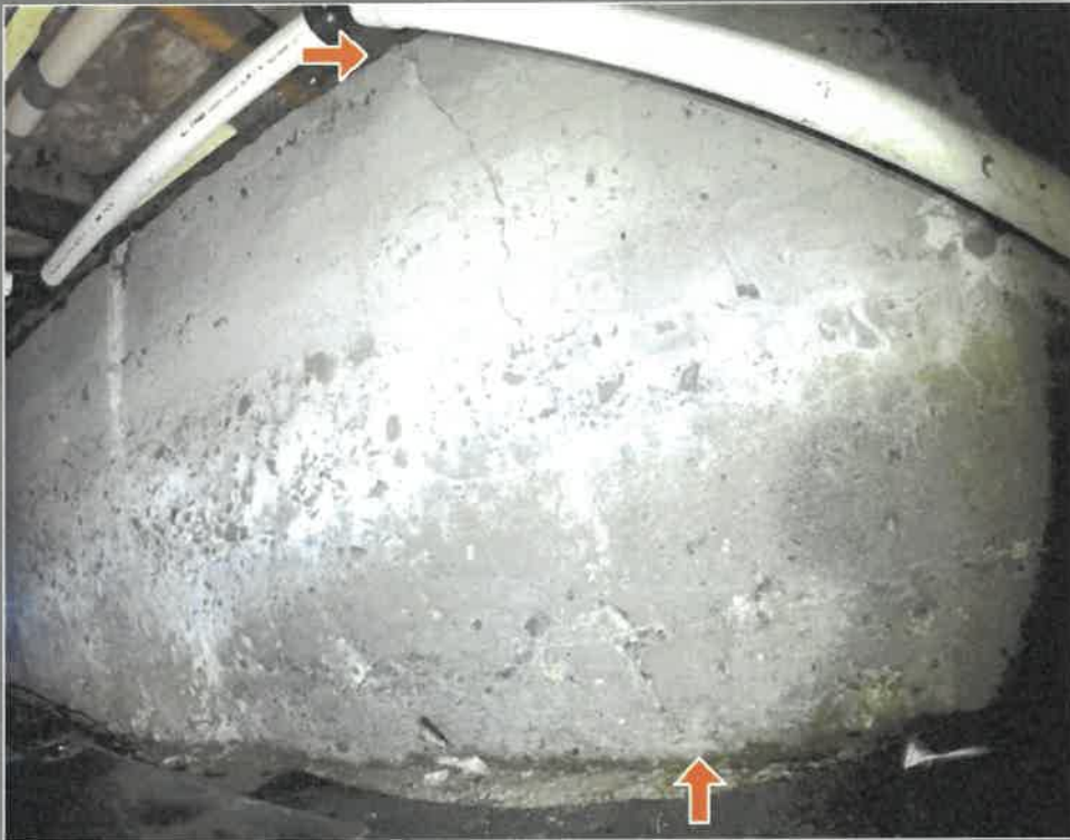
A. Item 3(Picture) Opposite side of crack in item 2
