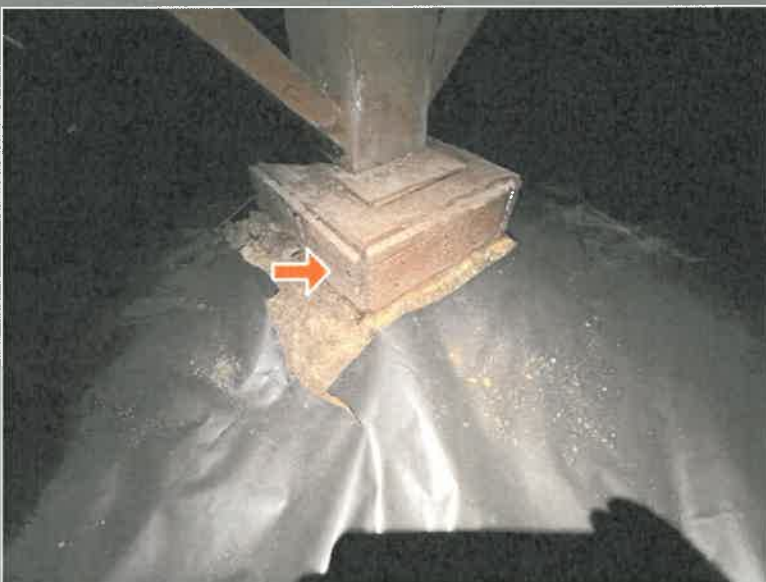
B. Item 20(Picture) Wooden forms left in place in contact with earth is perfect habitat for termites.
