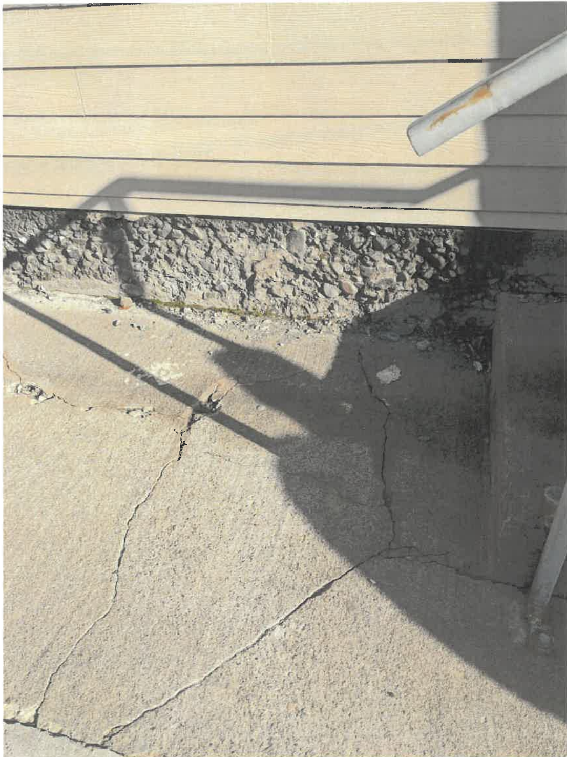
FIGURE 11: SCALING AND SPALLING AT FOUNDATION AT WEST SIDE OF STRUCTURE.
