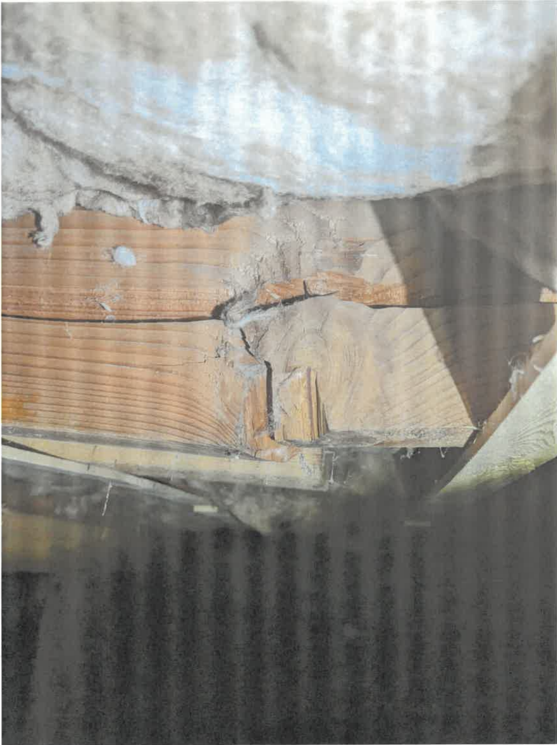
FIGURE 21: DAMAGED JOIST CAUSED BY KNOT IN HIGHLY STRESSED REGION. IT IS RECOMMENDED TO REINFORCE THIS JOIST AND/OR REPLACE.
