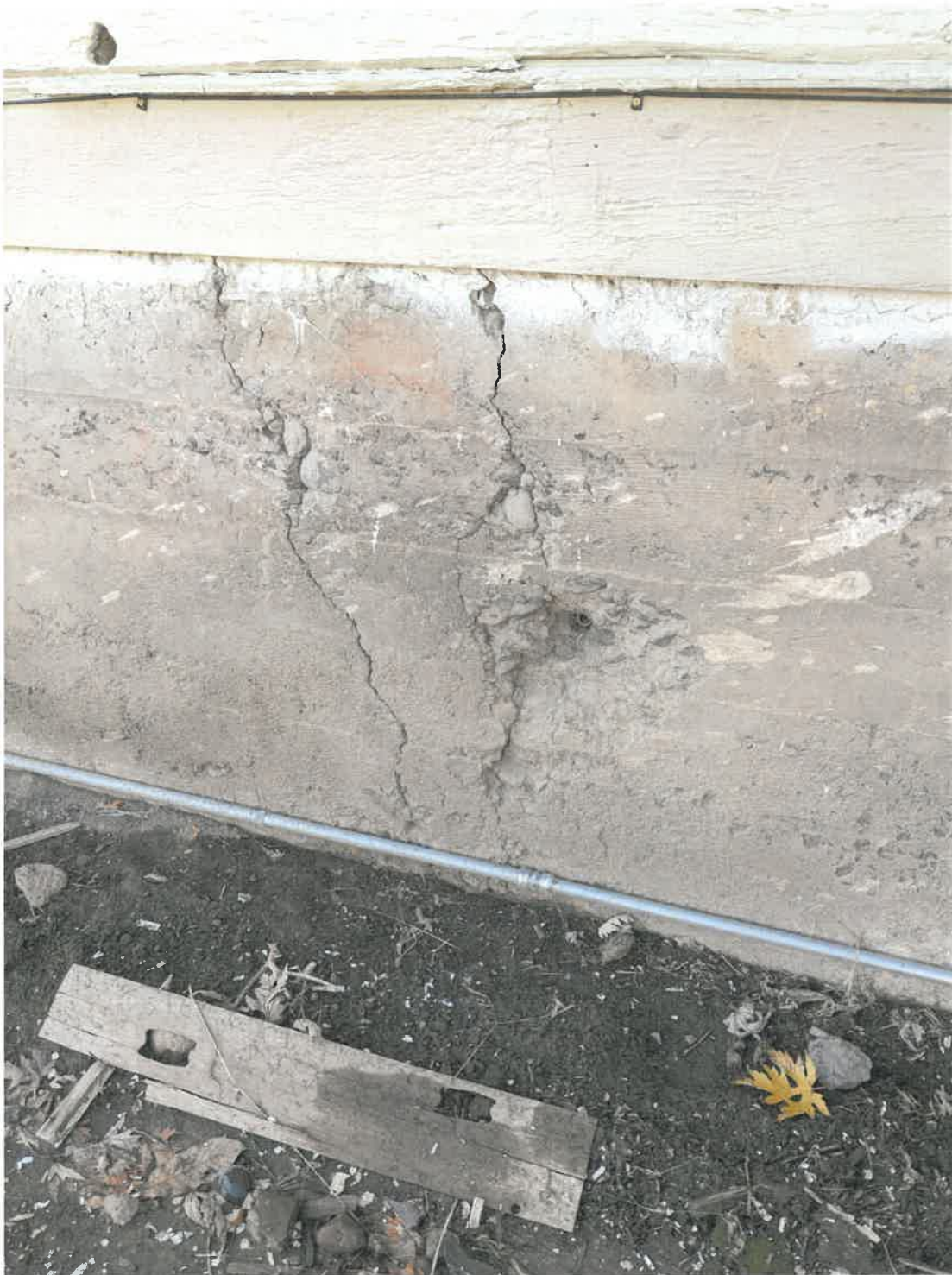
FIGURE 10: CLOSE UP AT POOR CONCRETE ON EAST SIDE OF STRUCTURE.
