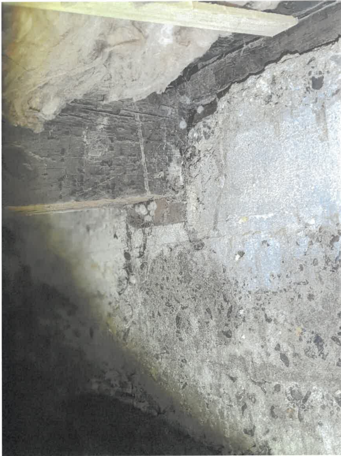
FIGURE 19: CHARRED AND FIRE-DAMAGED WOOD LEFT IN PLACE AT NORTH END OF STRUCTURE. THE RIM JOIST IS THE MOST SIGNIFICANTLY DAMAGED ELEMENT.
