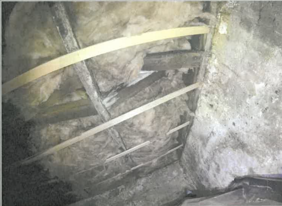
E. Item 3(Picture) Extensive decay found in crawlspace adjacent to sidewalk on cross bridging, joists and mudsill
