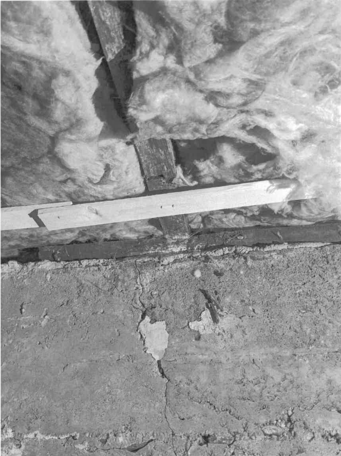
FIGURE 3: VERTICAL CRACKING ON INTERIOR FACE OF EAST FOUNDATION WALL. THE WOODEN JOIST AND SILL PLATE SHOW SEVERE DECAY AND ROT DUE TO MOISTURE, FURTHER SUGGESTING THAT VERTICAL CRACKING IS CAUSED BY MOISTURE.
